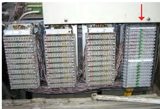
Expansion of a multifunctional enclosure fitted with a CH 80 for 100 twisted pairs to a CH 08HD for 200 twisted pairs, for the connection of active system technology.
